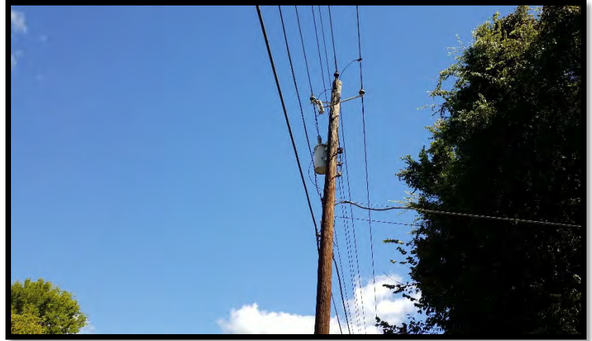
View of pole-mounted transformer near the boundary of PA-5.
