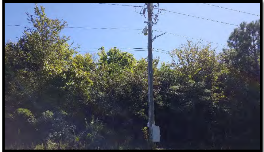
View of pole-mounted transformer on PA-2.
