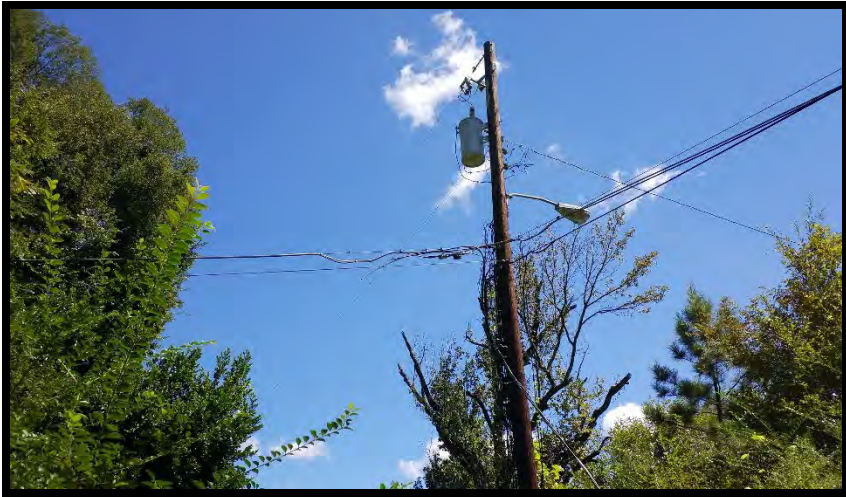
View of pole-mounted transformer on PA-5.
