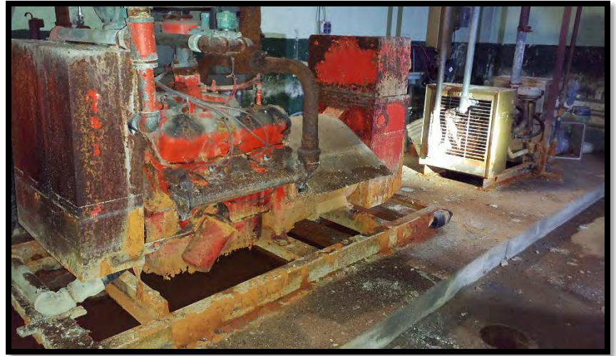
View of gas powered generator.
