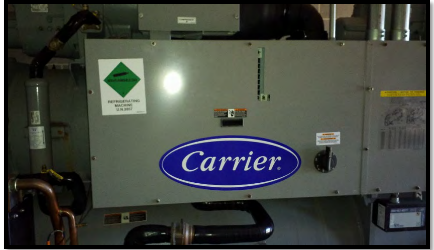
View of refrigerating machine in the small building.
