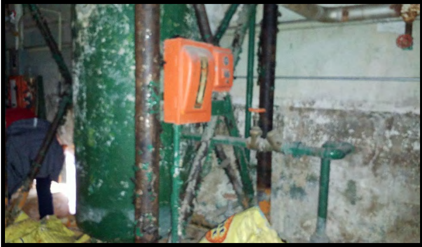
View of water softener tank.
