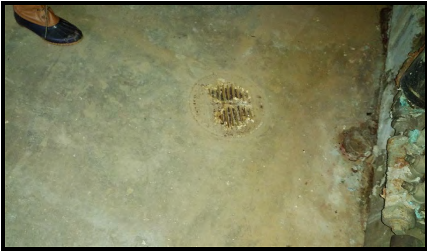
View of drain where chillers are located.
