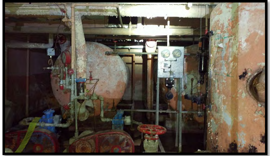
View of water tanks in basement.
