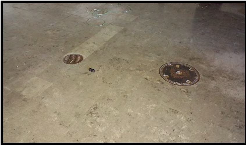
View of floor drain and manhole cover in room on ground floor.
