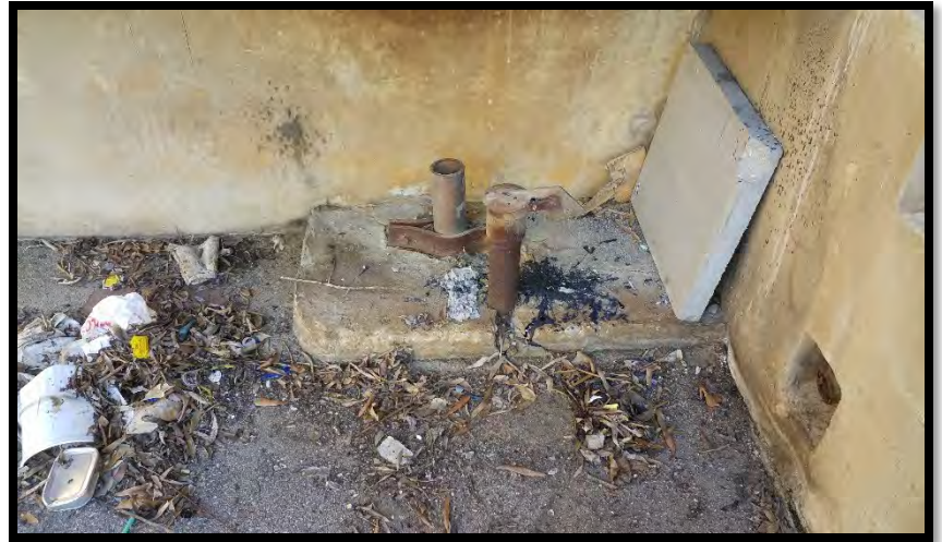
Exhaust pipe from natural gas generator.
