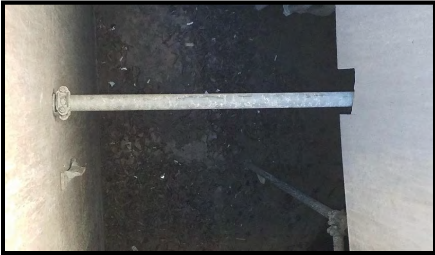
View of where transformers are contained.
