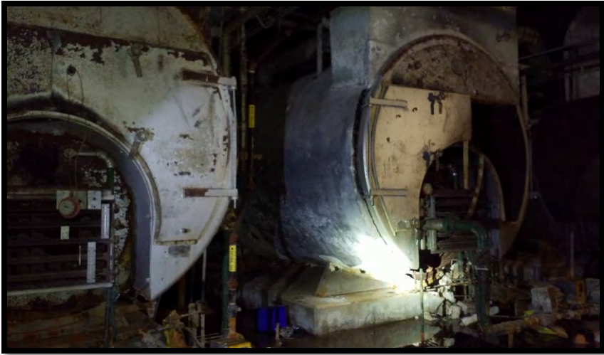
View of gas powered steam boilers.
