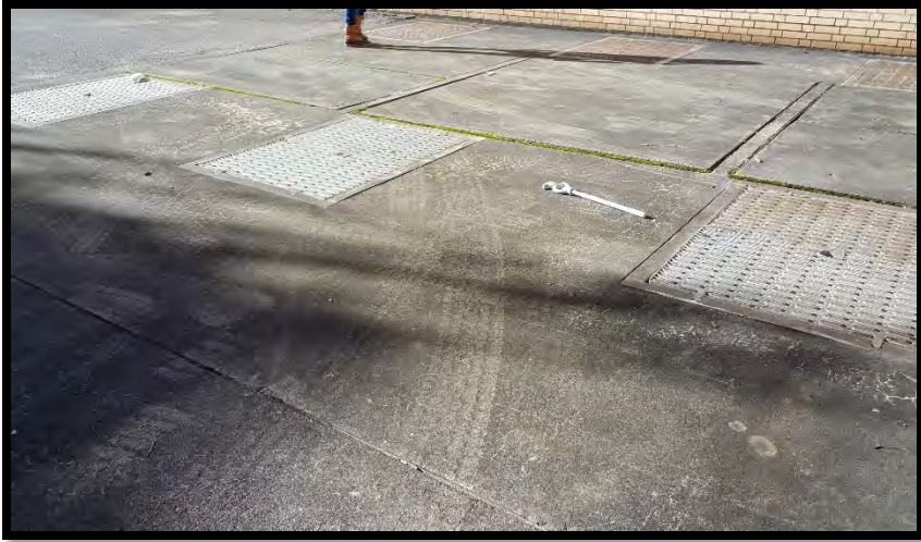
View of grates leading to transformers.
