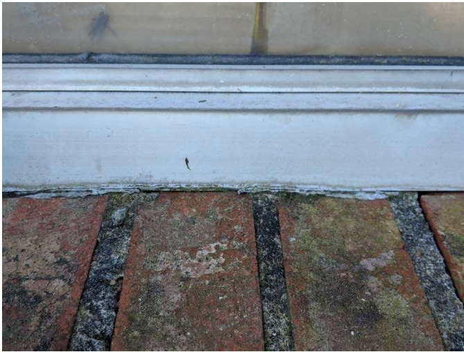
Photo #3 View of asbestos-containing gray caulk on metal windows & brick on exterior windows of office building
