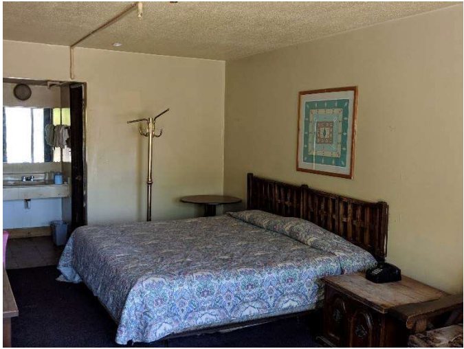
Photo #2 View of asbestos-containing ceiling texture in rooms 164-168 & 225-229
