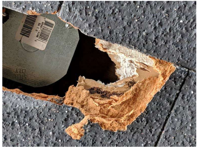
Photo #4 View of asbestos-containing texture and joint compound on non-asbestos drywall above non-asbestos 1'x1' ceiling tile
