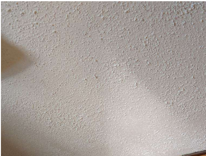
Photo 5 View of asbestos-containing ceiling texture in rooms 151-160 & 251-260
