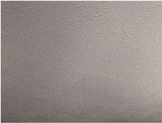
Photo #3 View of asbestos-containing ceiling texture in rooms 101-120 & 201-220
