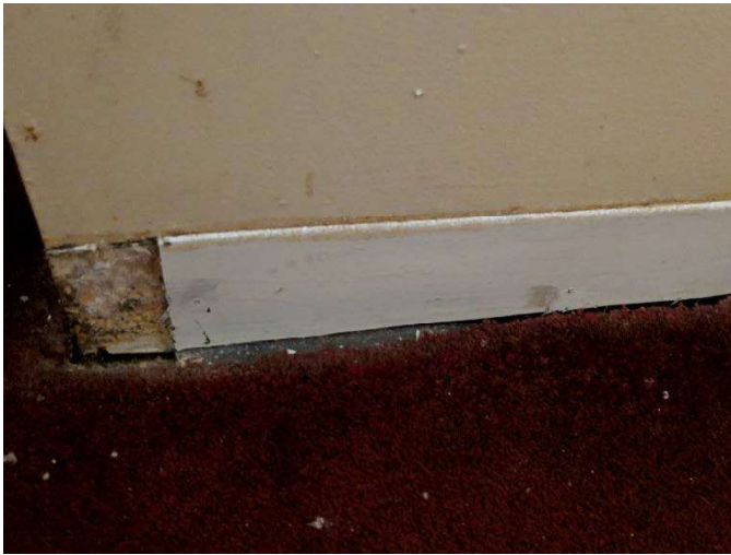
Photo 3 View of asbestos-containing joint compound on non-asbestos drywall in rooms 151-160 & 251-260
