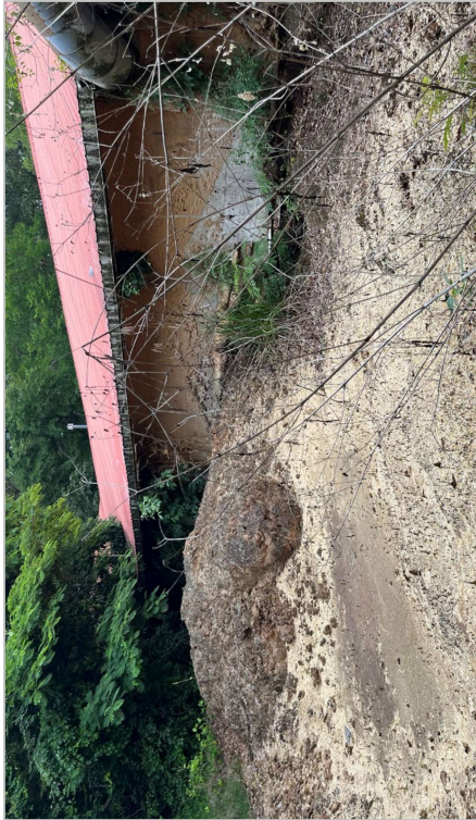
Sawdust and shavings pile along western exterior.
