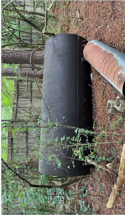
UST stored at rear shop exterior. Owner stated it came with building and was from offsite. No apparent evidence of spills or staining. Tank was empty and on side.
